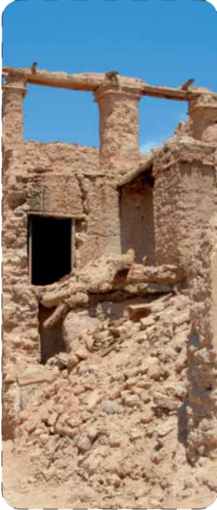
Observation of construction systems and pathologies
